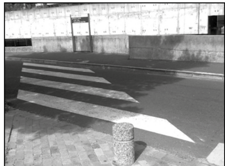
(f) Missing crossing facility kerb drops 6
