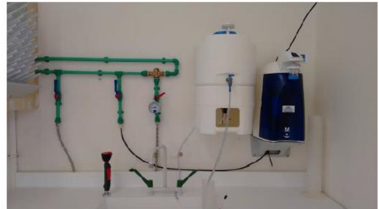
Water purification, thermostatic valve, flow restrictor and eye-wash station
