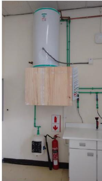
Geyser and Pressure pump (below)
