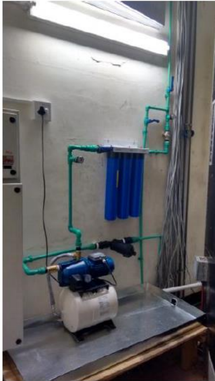
Pre-filtration and booster pump (in corridor)
