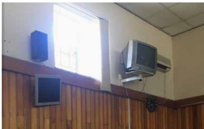
Figure 5: Old and broken CCTV Cameras in a Rural Court
